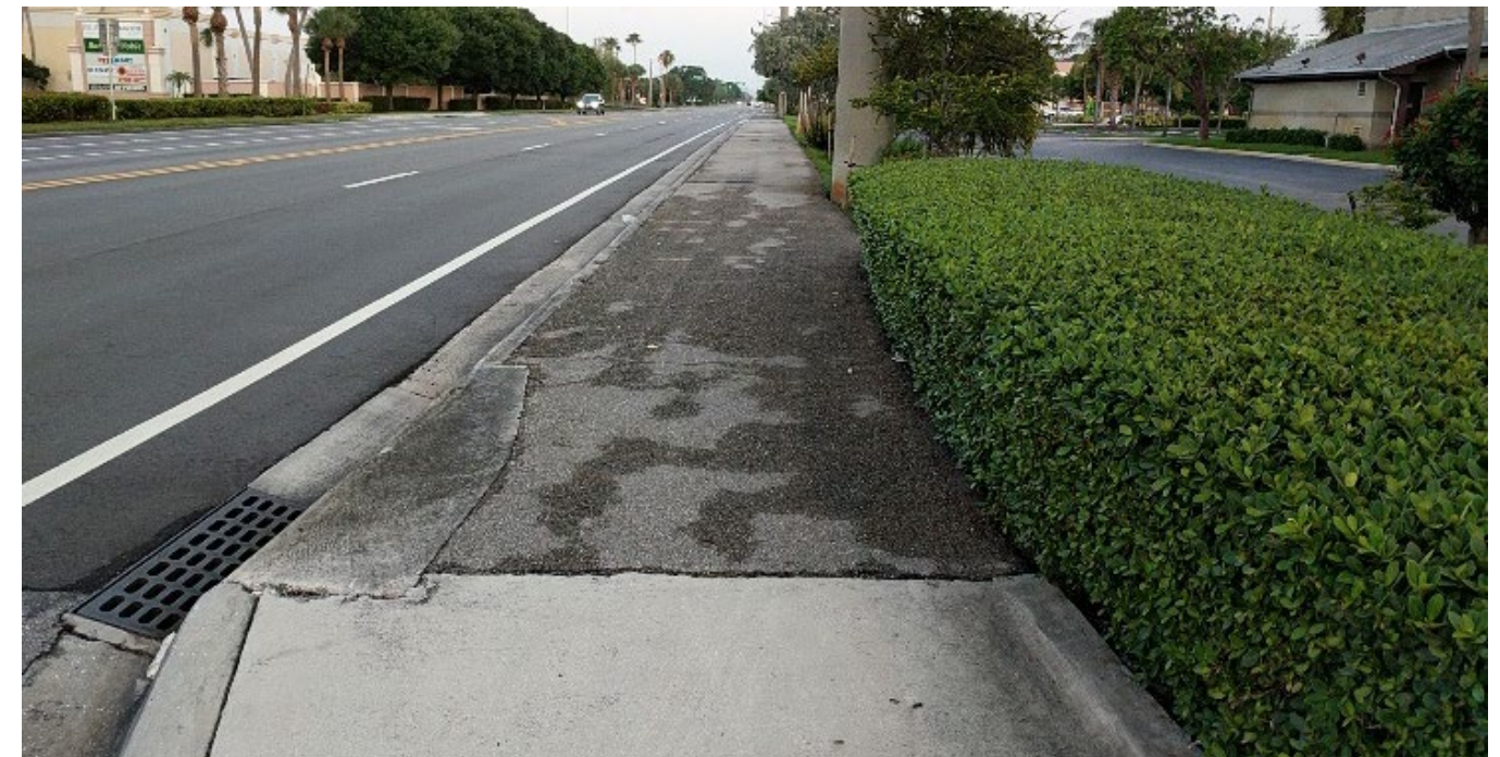
8 ft sidewalk North of Boynton Beach Blvd on N. Congress; Photo by: CTS Engineering, Inc.
