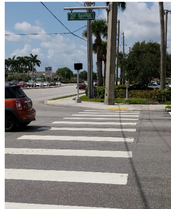
Signalization not working at intersection of Old Boynton and Congress; Photo by: CTS Engineering
