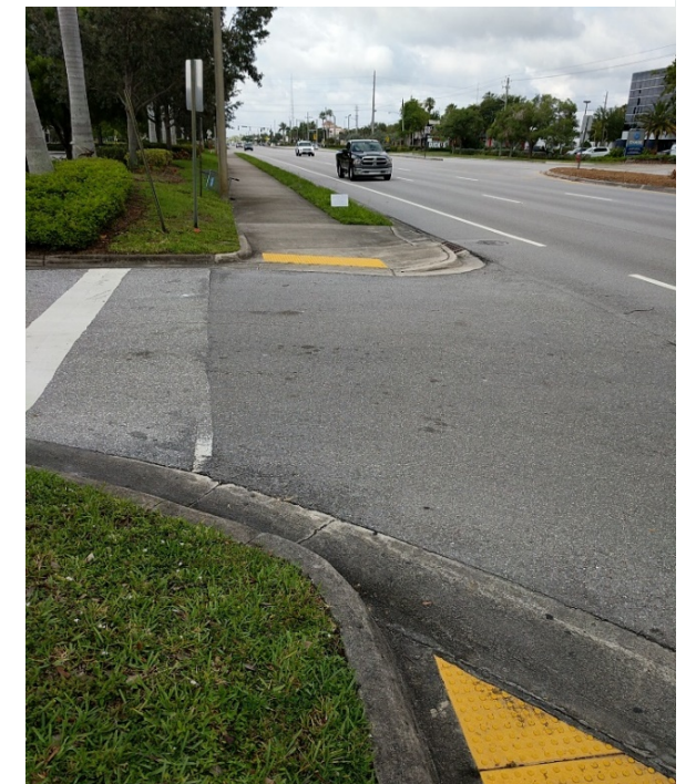
Crosswalk needed on Congress, North of Old Boynton; Photo by: CTS Engineering, Inc.
