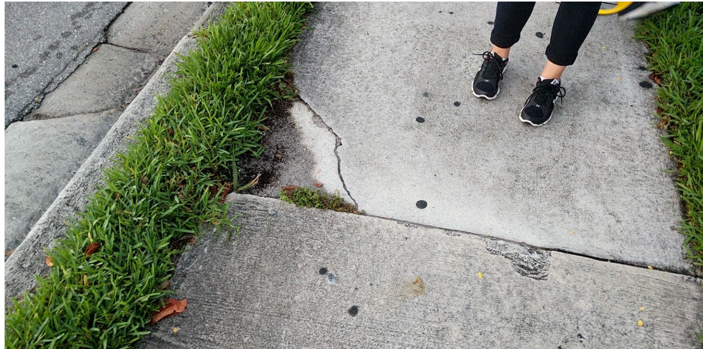
Broken sidewalk along corridor near Old Boynton and N. Congress; Photo by: CTS Engineering, Inc.
