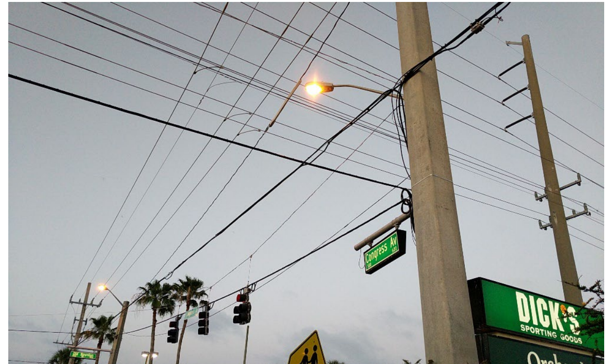
Lighting at intersection of N. Congress and Old Boynton; Photo by: CTS Engineering, Inc.
